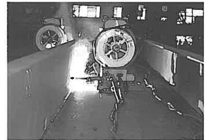
Fig.4 Fillet welding of longitudinal components by using a portable fillet welding carriage and MX-200 in shipbuilding (By courtesy of Tsuneishi Shipyard, Japan)
