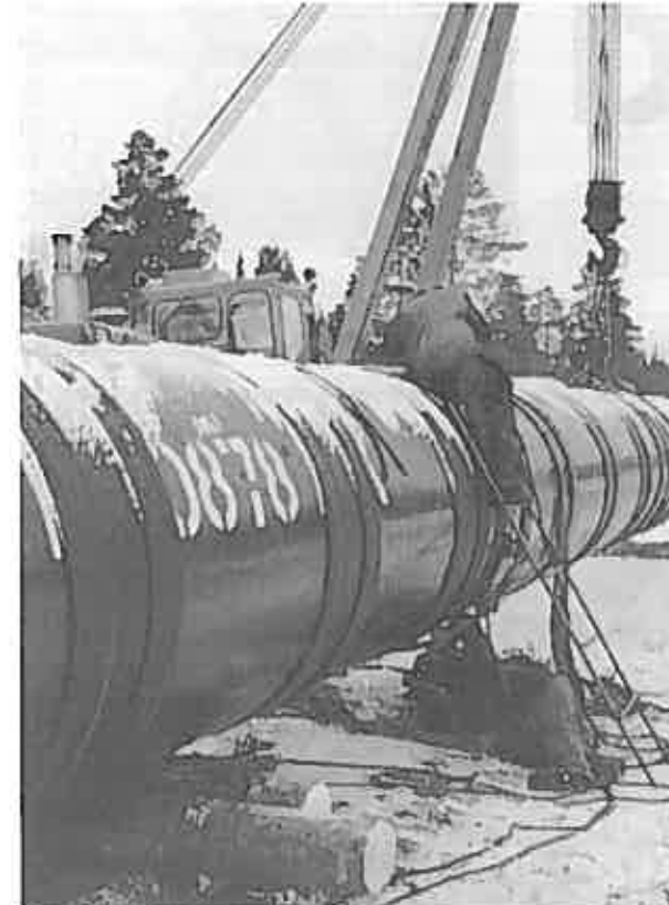
Fig. 3 - A pipeline-welding site in Russia where LB-52U is used for joining the girth joints in freezing weather
