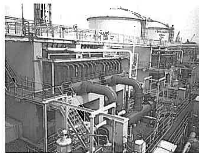
Fig. 3 - Cooling piping of the energy plants is one of the applications of NC-36L because of superior pitting corrosion resistibility against chloride ions.
