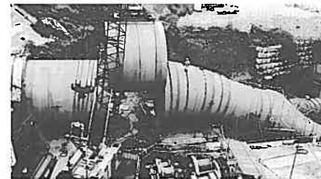
Fig. 3 - The construction of penstocks for hydraulic power generation requires the welding procedures be strictly controlled, because the welding circumstances are very severe in terms of humid welding atmosphere, and confined welding spaces.
